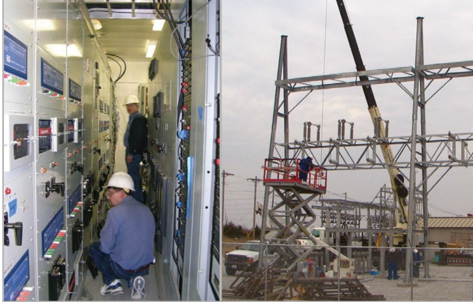
(Left) Inspecting new relay panels (Right) Houston #2 Substation major rebuild
