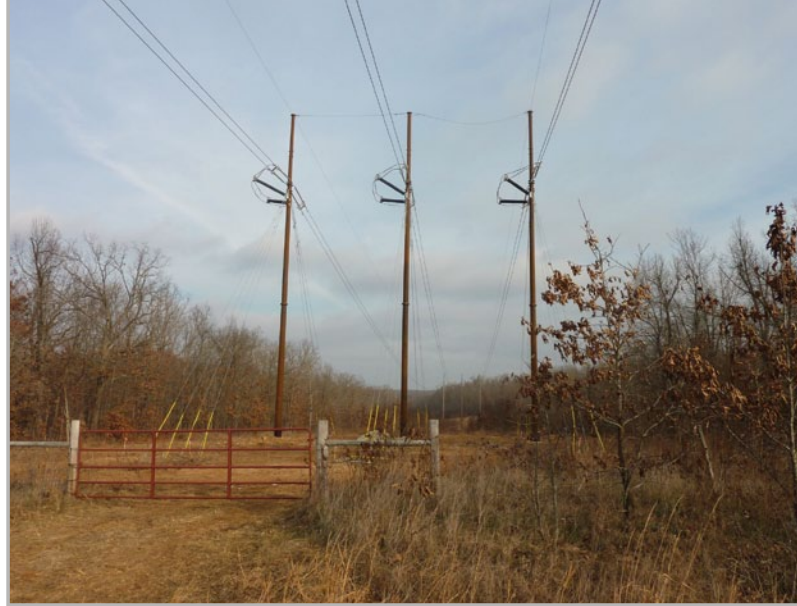
Typical 345 kV Storm Structure
