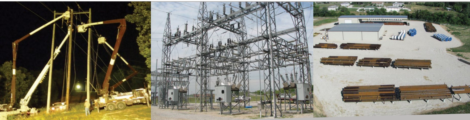
(Left) Planned night outage work on the Mansfield to Hartville line (Center) New breaker installation at Ava #2 (Right) 345 kV Emergency Material Yard
