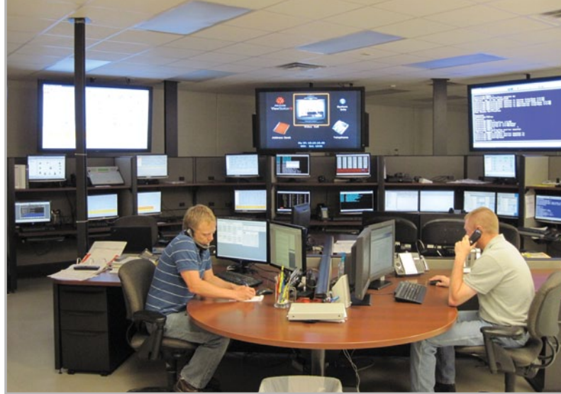
The Network Operations Center
